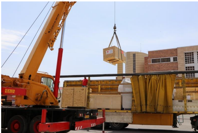
Fig. 7. Unloading of MRI machine at Kousar hospital in Semnan, Semnan Province. © WCO Iran
